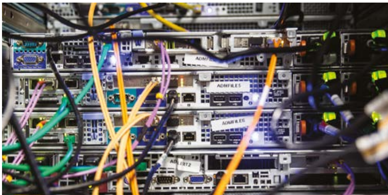
Datacenter Ecole Polytechnique © EcolePolytechnique J.Barande
